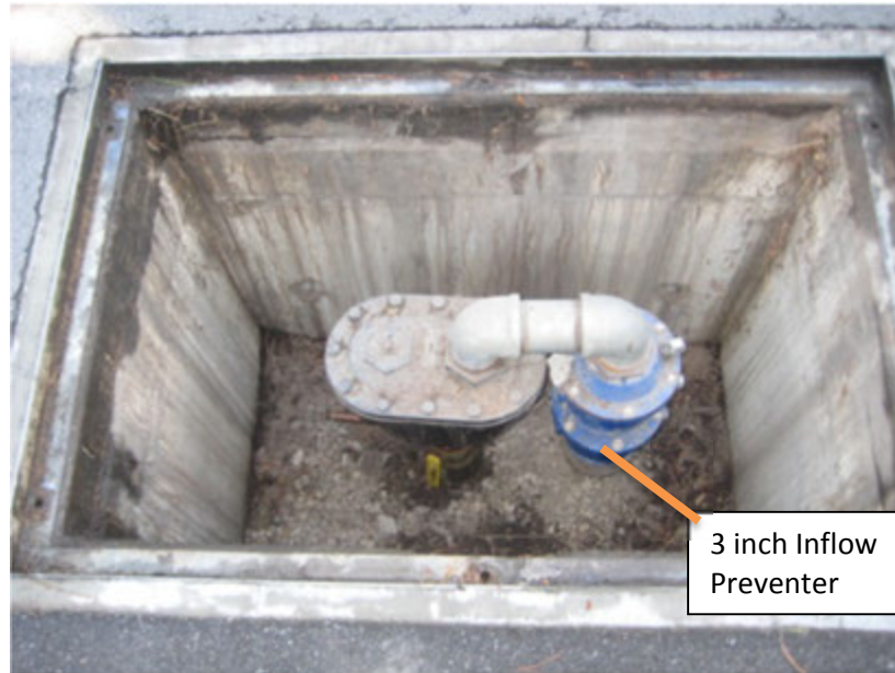
FIGURE 6. Air Valve Vault, Foster City, CA
